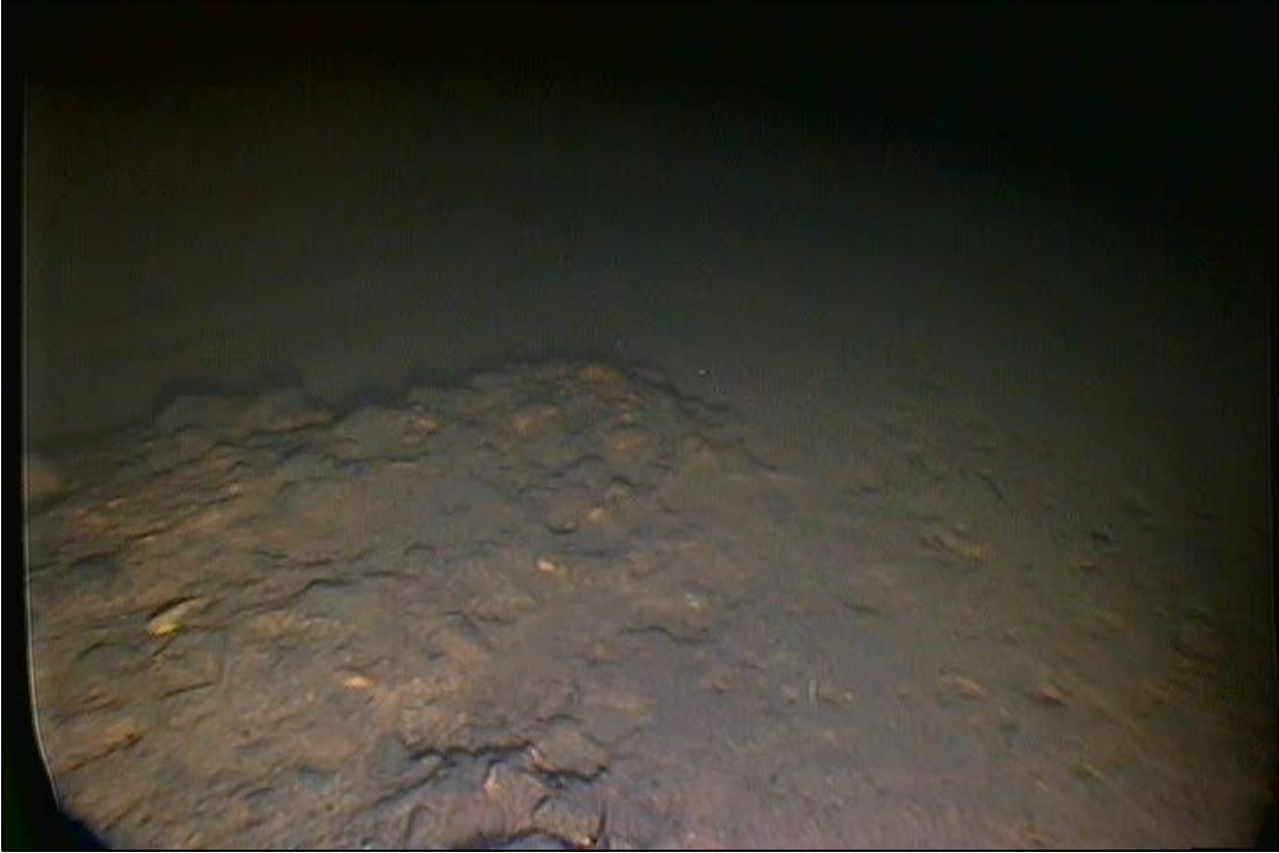
Figure 4 Images of apron erosion in area just upstream of baffle blocks in Bay 18.
