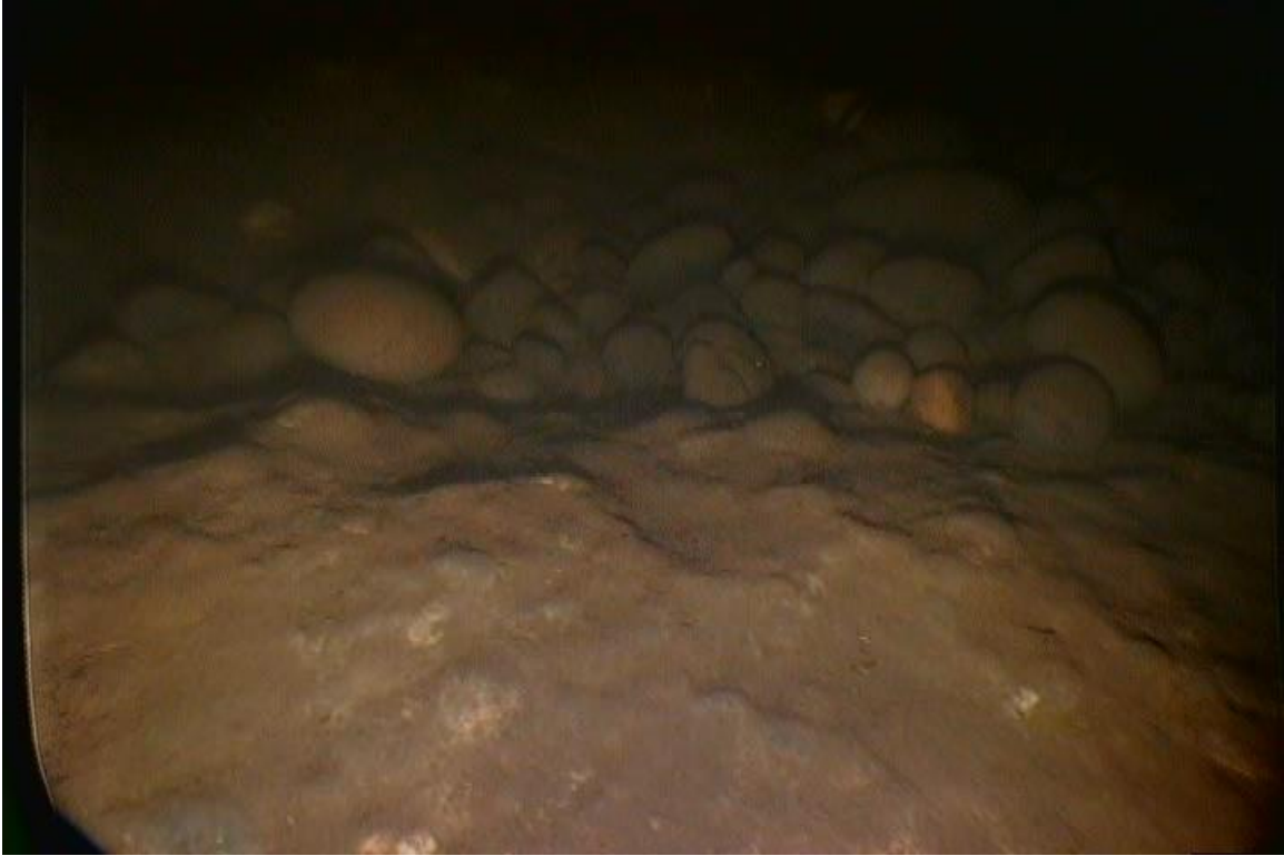
Figure 3 Bay 17 eroded area filled in with rock.
