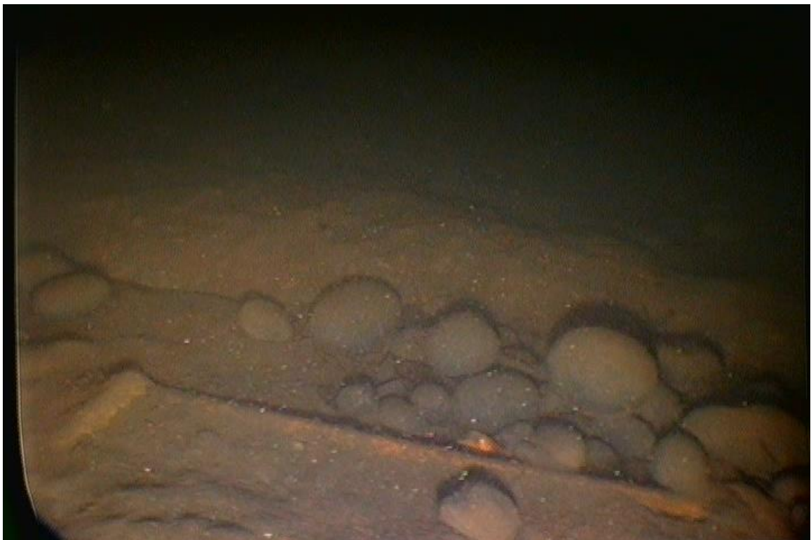
Figure 9 Bay 17 erosion and exposed rebar.
