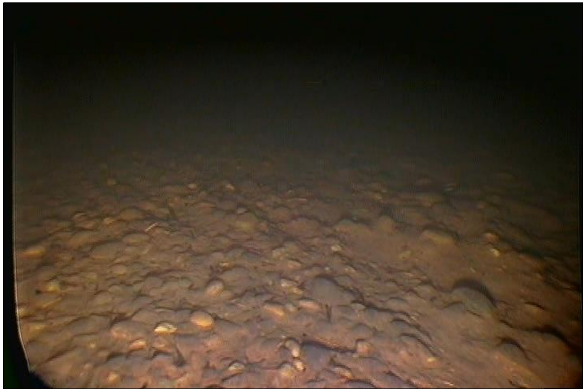
Figure 13 Additional image of Bay 18 erosion at base of the ogee.
