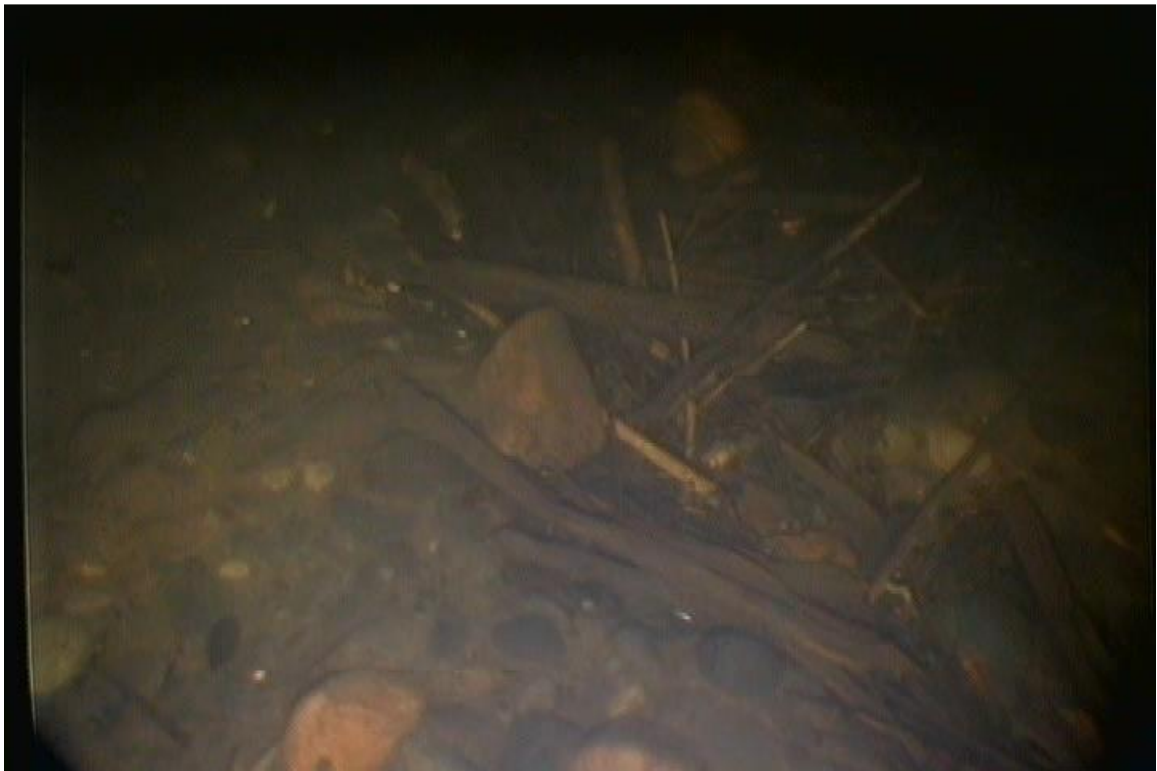
Figure 17 Woody debris in eroded area of Bay 18 ogee.
